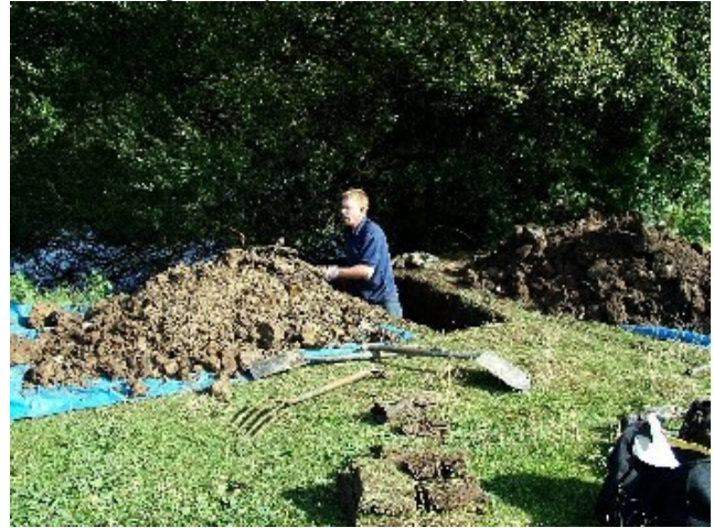
Photo 4. Darren in the test trench on the first day bounded by separate tarps for topsoil and tip contents
