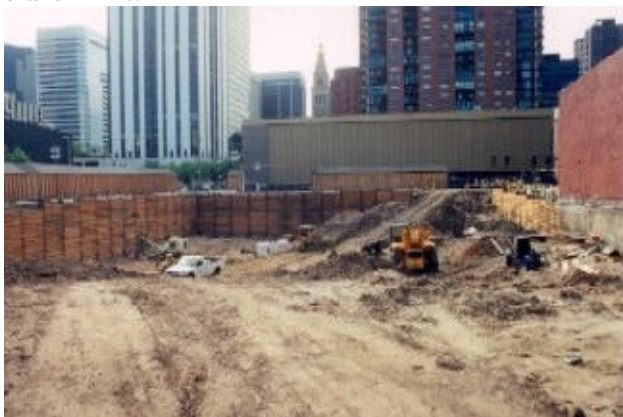
In the background of the picture of the construction site is the ramp along which we found the privy for the Clark, Gruber & Co. and Denver Branch of the U.S. Mint.
